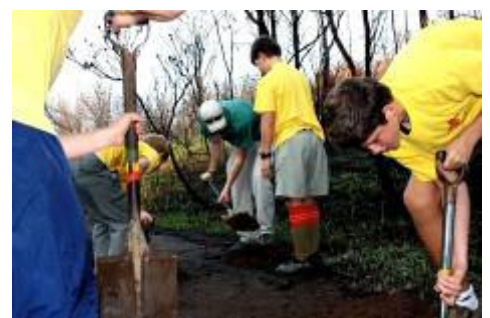
Scouts hard at work repairing the boardwalk under the supervision of Robert Le Brun, conservation student.
